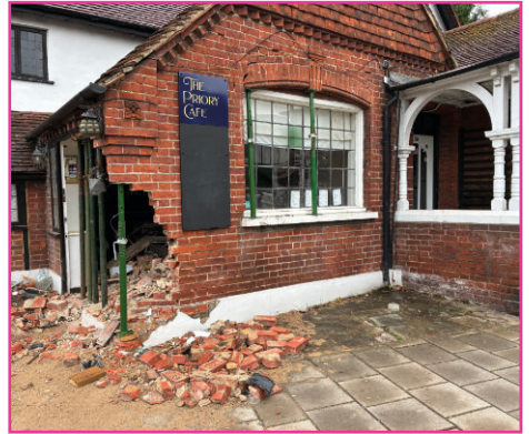
Damage to the Priory Café
